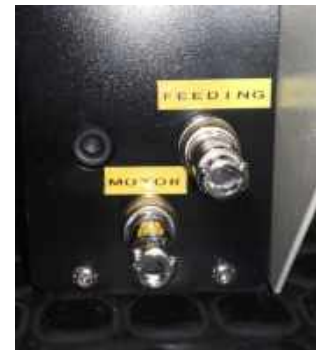
External screw distribution control by PLC
